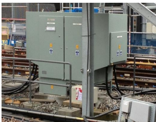
Figure 18 – Trial Slave Contactor located adjacent to the IRJs used for AC / DC interface separation
