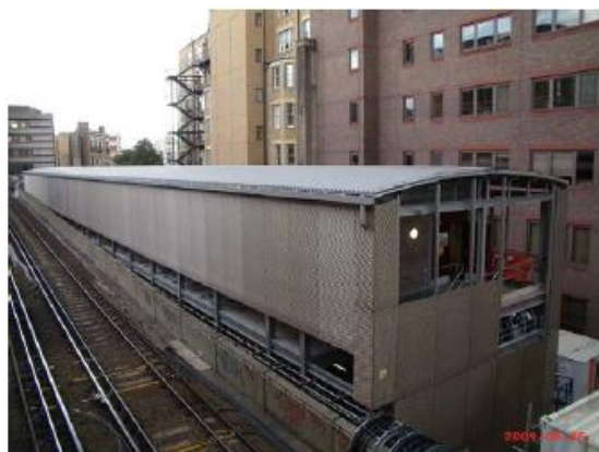
Figure 10 – Ludgate Cellars combined AC / DC interface and DC traction substation
