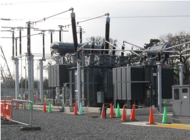
Figure 3 – One of the National Grid transformers at Elstree required to support the AT system
