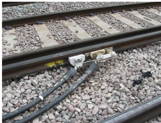
Figure 7 – Typical ETE works showing upgraded hookswitch
