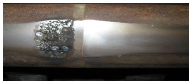
Figure 16 – Typical example of IRJ rail head arcing
